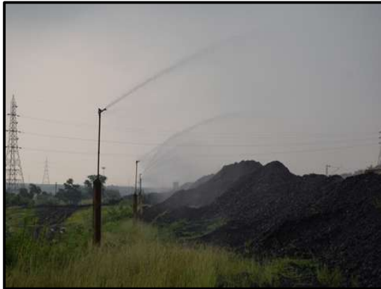
Fixed sprinklers at Belpahar Coal siding
